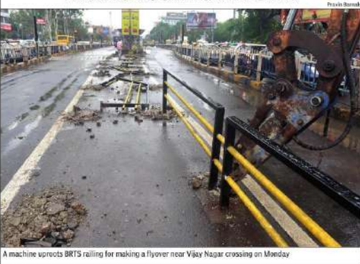
A machine uproots BRTS railing for making a flyover near Vijay Nagar crossing on Monday
